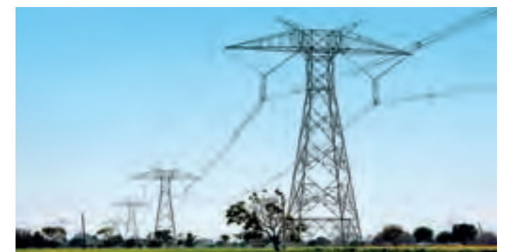
800 kV transmission lines between Nidhura and Agra.
