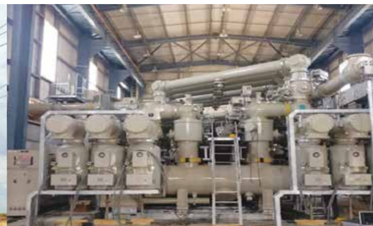
765 kV Gas-insulated Substation, Nizamabad, Telangana
