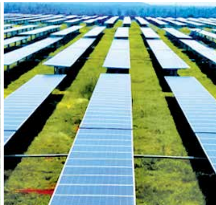
22 MWp HFE Solar PV, Karnataka
