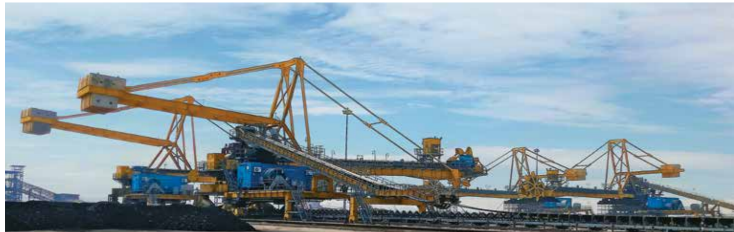
Bucket Wheel Stacker Reclaimers at Adani Dhamra Port – DPCL
