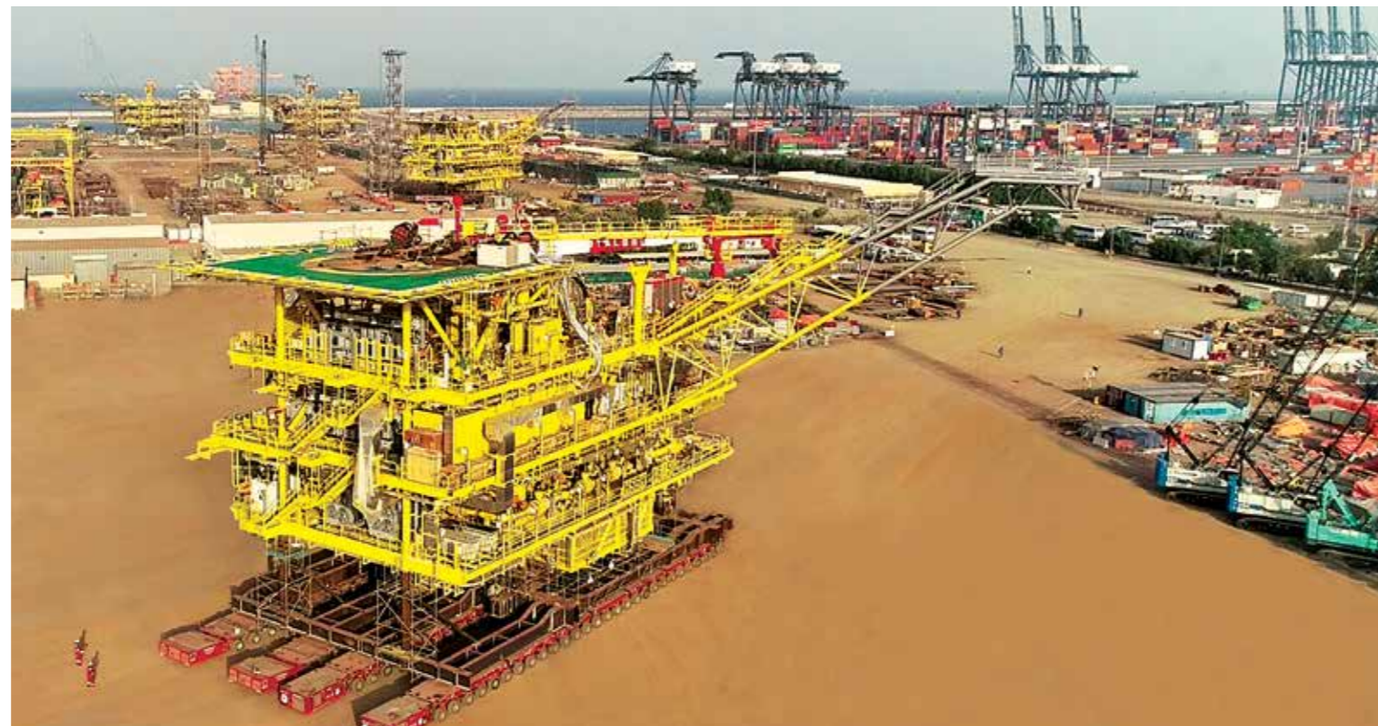
Six Gas Production Modules and two mega Tie-in Platforms (7000 MT each) for Hasbah II fabricated at LTHE's Oman Facility
