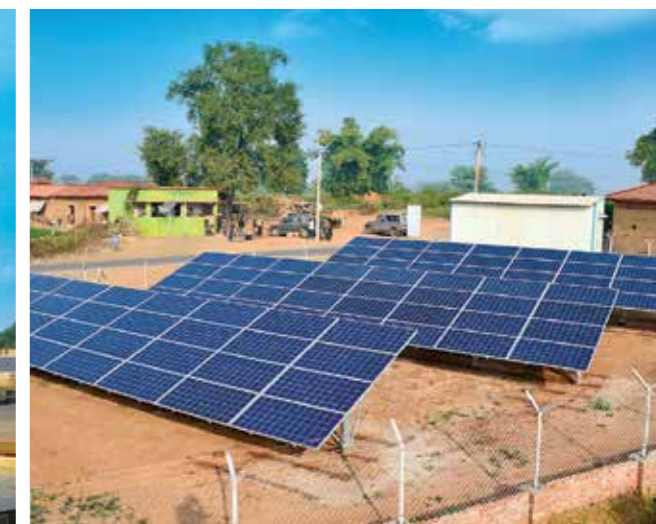
Micro-grid Project for Rural Electrification in Bihar
