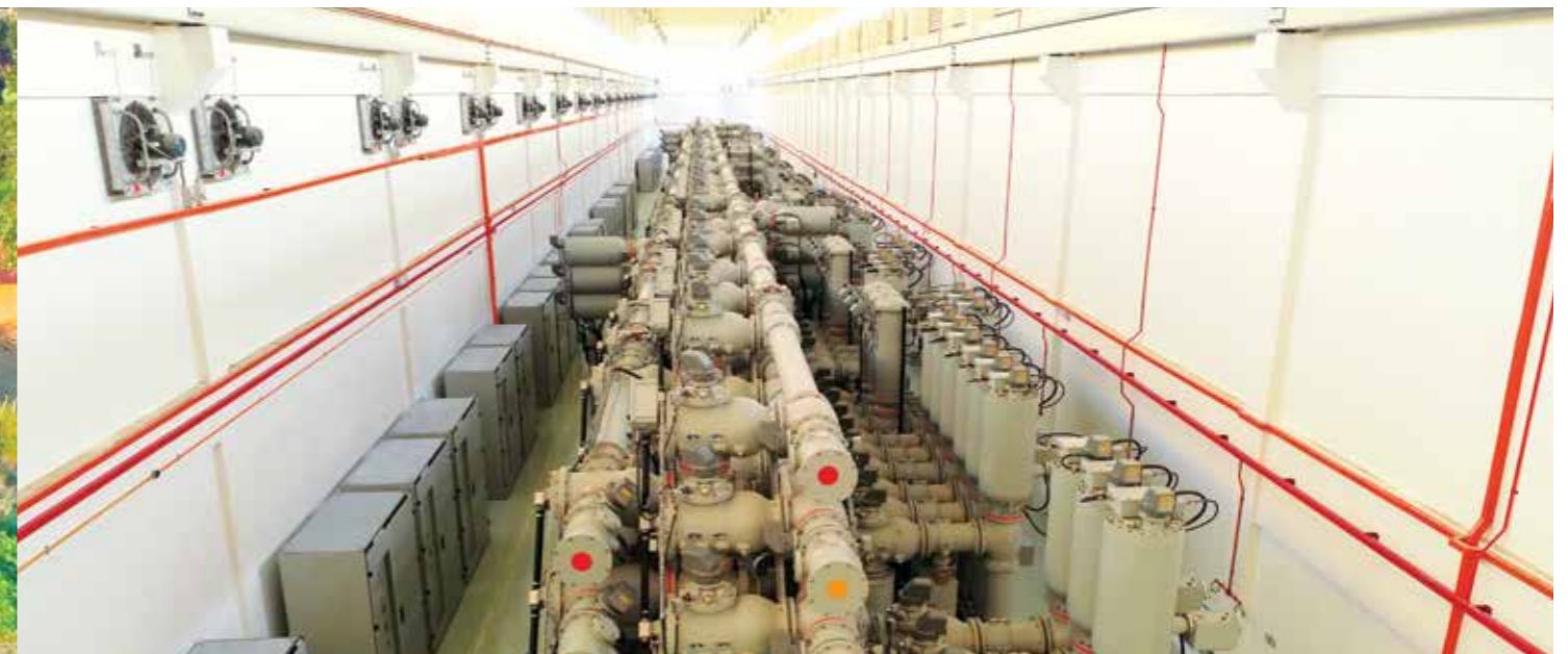
Lambir 275/132-33 kV Gas-insulated Substation, Sarawak, Malaysia
