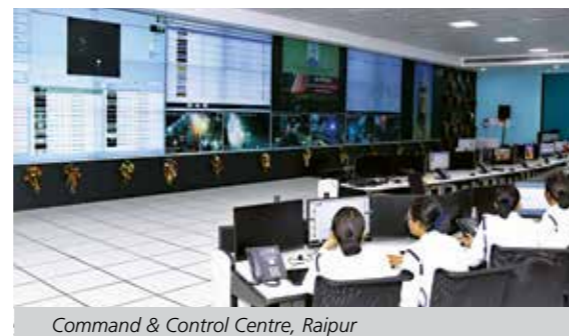
Command & Control Centre, Raipur
