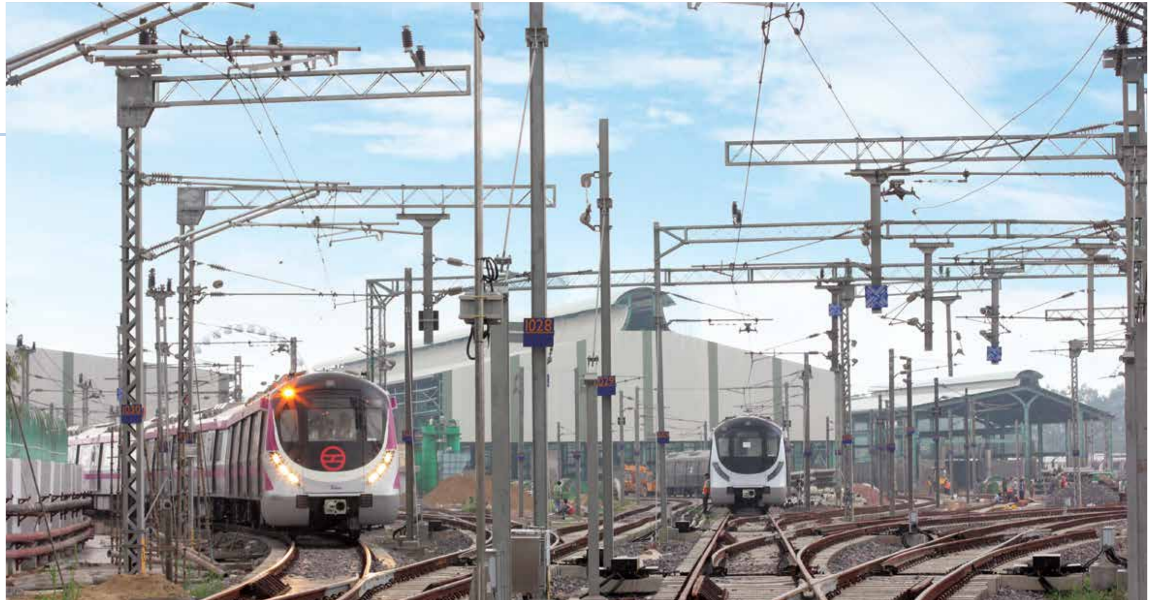
Overhead Electrification for Delhi Metro
