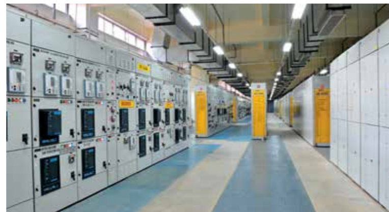
Control Panels at MRPL
