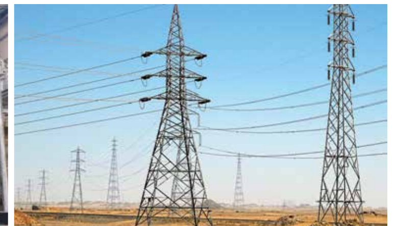
Toshka 2 – Wadi Halfa 220 kV Transmission Line, Egypt
