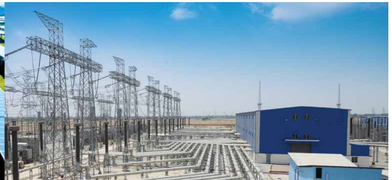
765 kV Gas-insulated Substation, Varanasi, Uttar Pradesh
