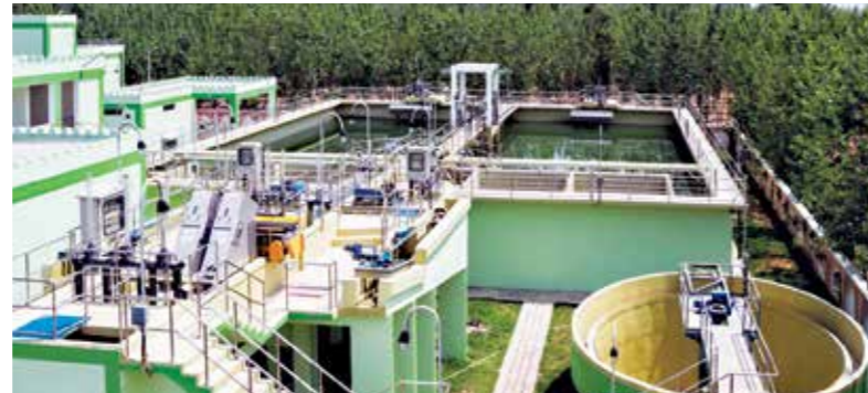
5 MLD Sewage Treatment Plant, Rampur, Uttar Pradesh
