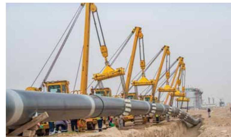
48" x 118 km-long Crude Transit Line from North Kuwait to Central Mixing Manifold for KOC
