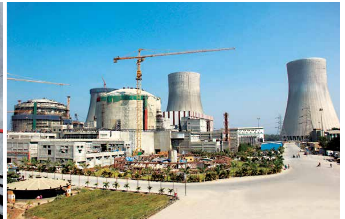
Kakrapar Atomic Power Plant under construction. L&T has been associated with almost all of India's nuclear power plants.
