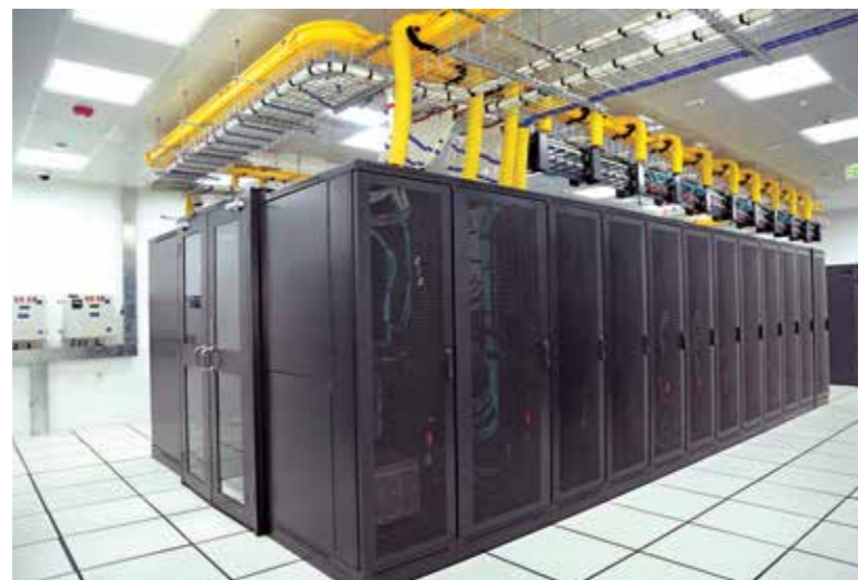
Data Centre for Hyderabad Safe & Smart City
