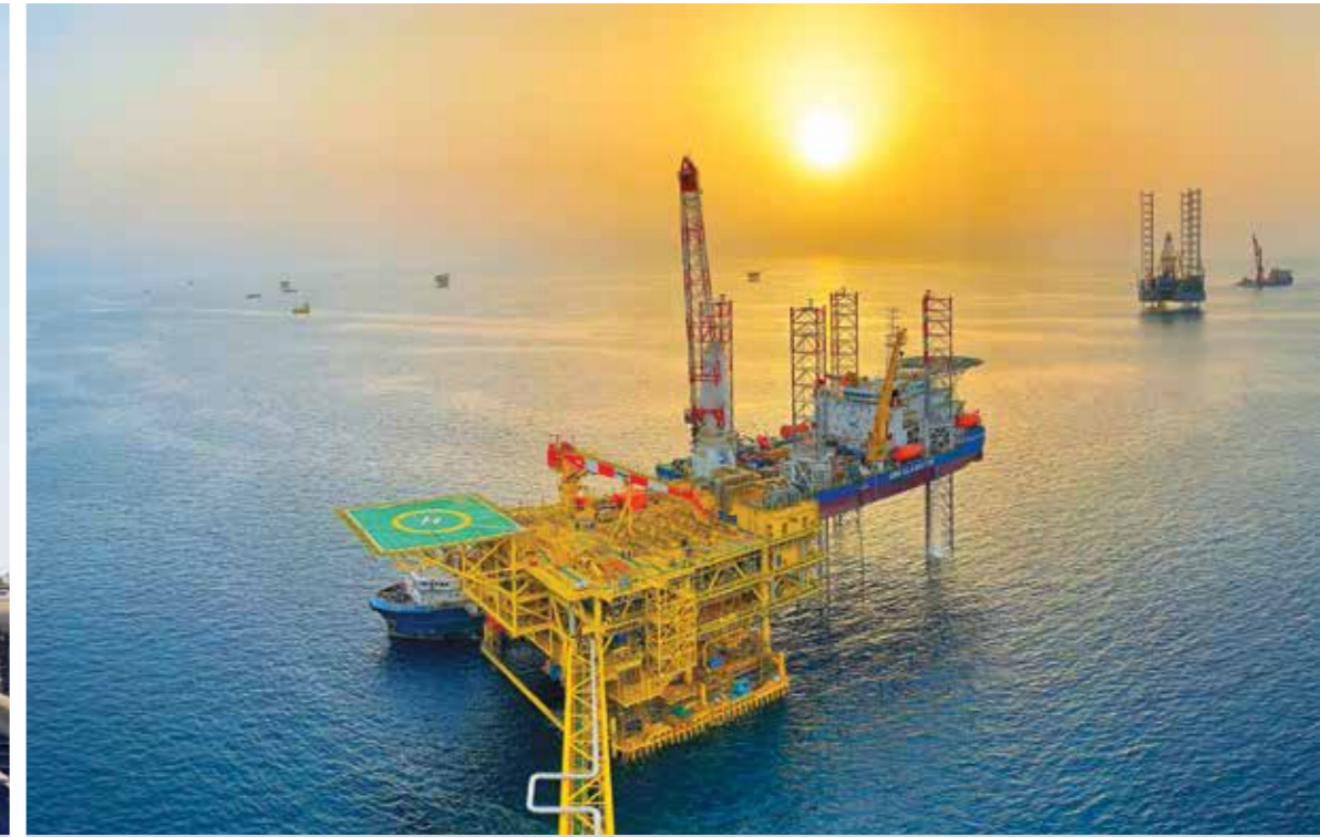
The heaviest, fully integrated gas platform in Saudi Aramco's history, installed by float-over method for Hasbah II
