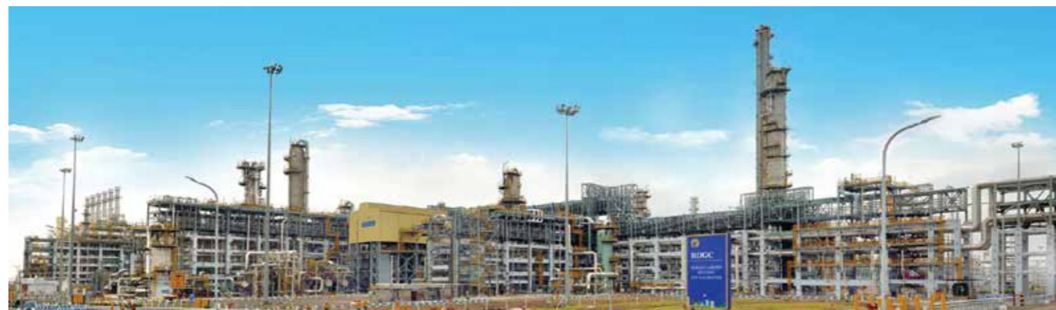
Construction of the world's largest Pet Coke Gasification Complex and Refinery Off Gas Cracker for Reliance Industries at Jamnagar, India
