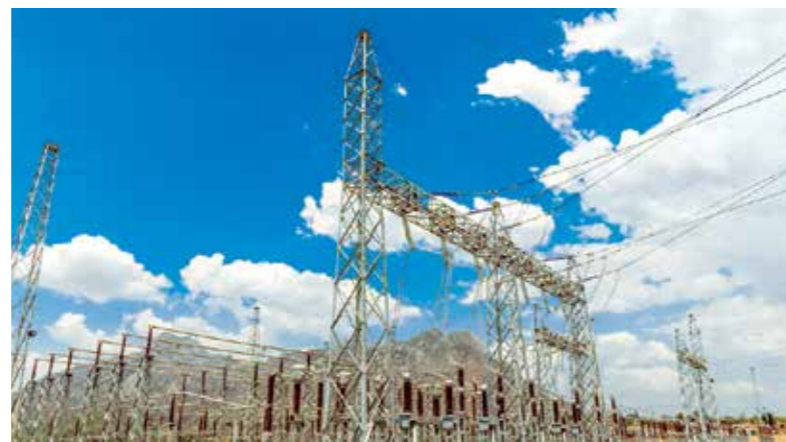
400/132 kV Substation, Nkhoma, Malawi
